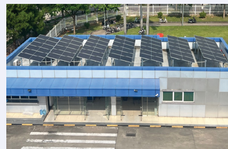
▲ Solar Modules at the Vietnam Manufacturing Subsidiary
