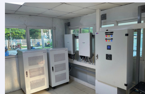
▲ Energy Storage System(ESS) at the Vietnam Manufacturing Subsidiary
